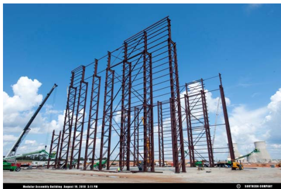
Modular Assembly Building, Aug 2010
